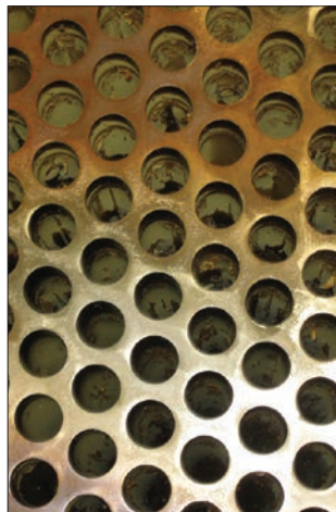
Figure 1. Evaporator tube appearance prior to hydro-blasting after treatment with Buckman anti-scale.
