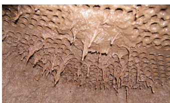
Untreated generator transformer oil cooler
