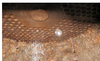
Treated generator transformer oil cooler
